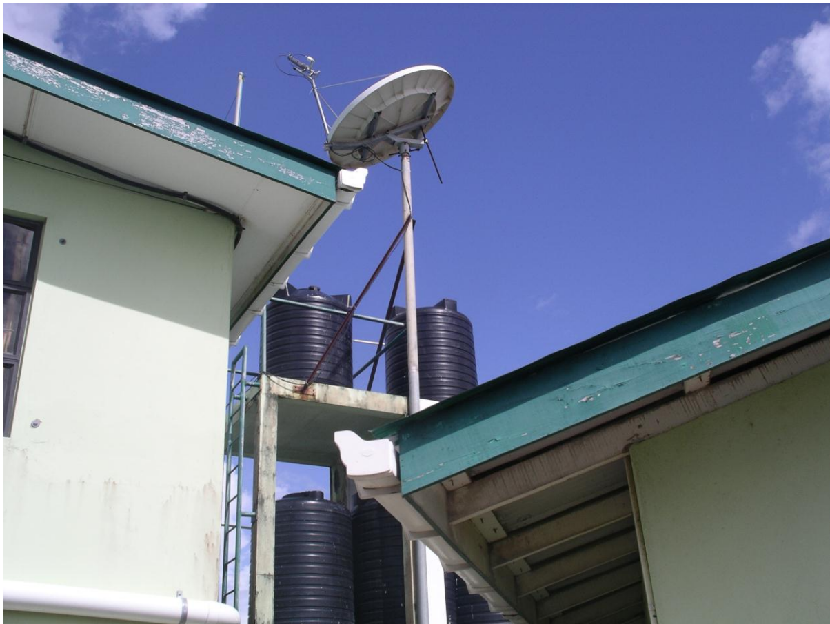
Wireless satellite receiving dish for the WAN at GFC Headquarters
