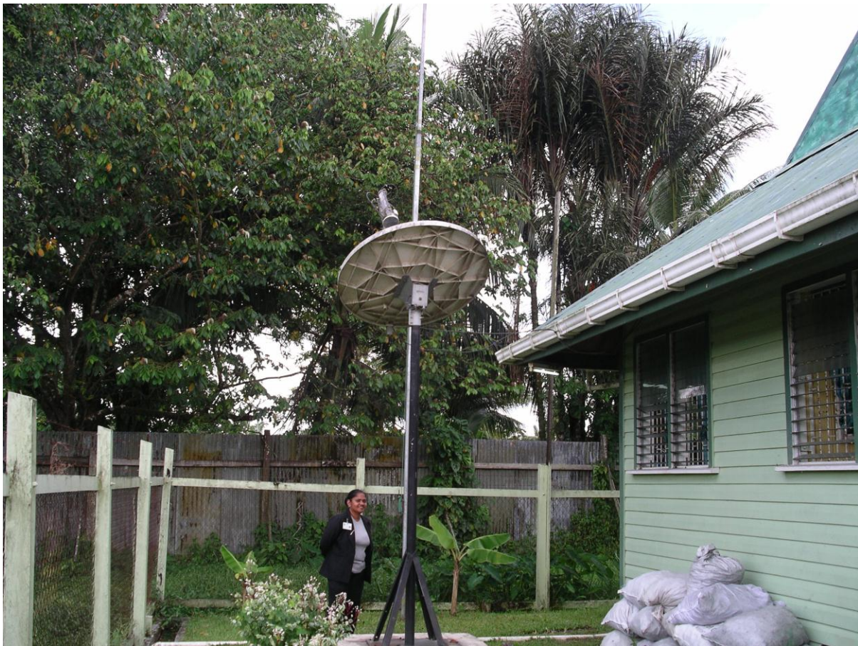
Satellite Dish at the Soesdyke Checking Station for accessing data from the central database at Georgetown.
