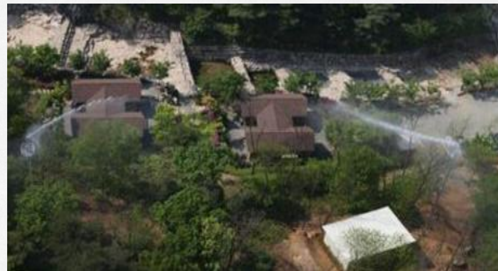
Forest Fire Extinguishing Facilities
