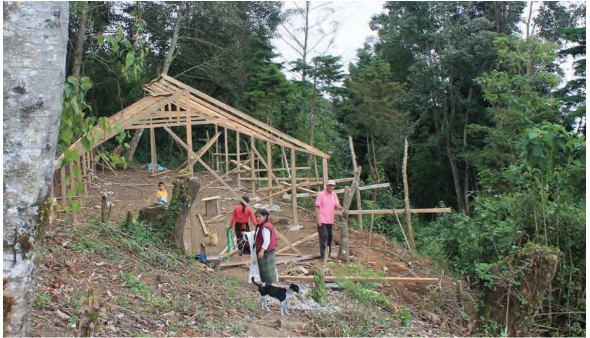
Budding enterprise: Villagers construct a greenhouse for growing roses for commercial sale as part of project activities aimed at increasing incomes for local people. Photo: Edgar Pérez/HELVETAS
