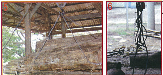
Figures 5-6. Log craning using damaged steel chain and steel cable
