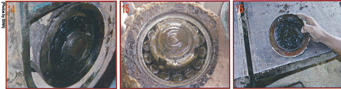
Figures 14-16. Improper greasing of band wheel bearing: late greasing (14), incorrect application of grease (15) and use of low speed grease (16)
