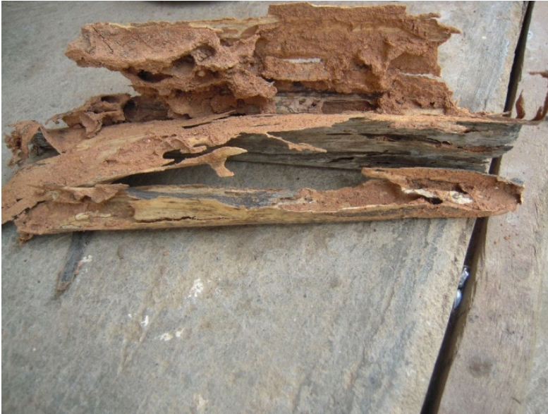
Fig.9.4b: Termite attack and damage of wood
