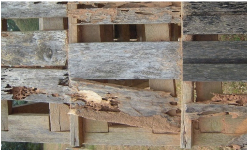
Fig.9.4a: Termite attack and damage of wood
