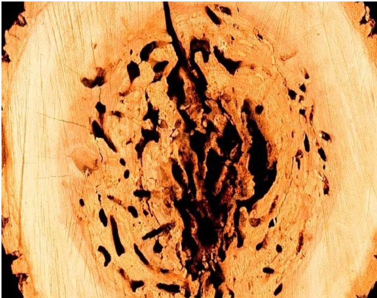
Fig. 9.5: Carpenter ant attack and damage
