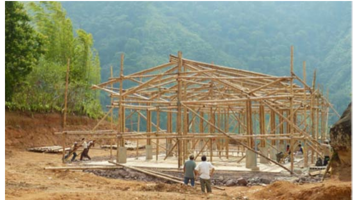
Learning by doing: Local capacity building included community training in house construction techniques as part of a program to build MINCABAMBÚ.
