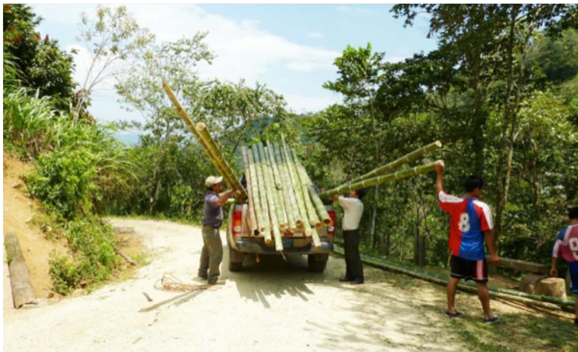
Vegetable steel: Workers load recently harvested bamboo onto a truck for transport to a construction site in Aramango District, Amazonas, Peru. Photo: J. Takahashi, PERUBAMBÚ
