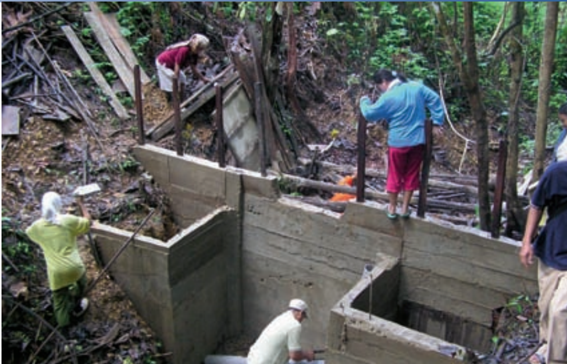
Concrete action: Longhouse members work with project staff to construct a valley pond. Photo: S. Lanjang
